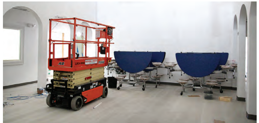
The Boys & Girls Club of the Northern Neck recently began construction of a new 10,000-square-foot Youth and Teen Activity Center at 8200 Northumberland Highway in Heathsville. Phase 1 of the $4.4 million project includes this dining center along with an art space, STEM lab, teen area and learning center. Work should be completed in the spring. Construction of Phase 2, which includes a 9,000-square-foot gymnasium and multi-purpose space, will begin this summer. Architectural work was done by GuernseyTingle with construction by Henderson, Inc.
