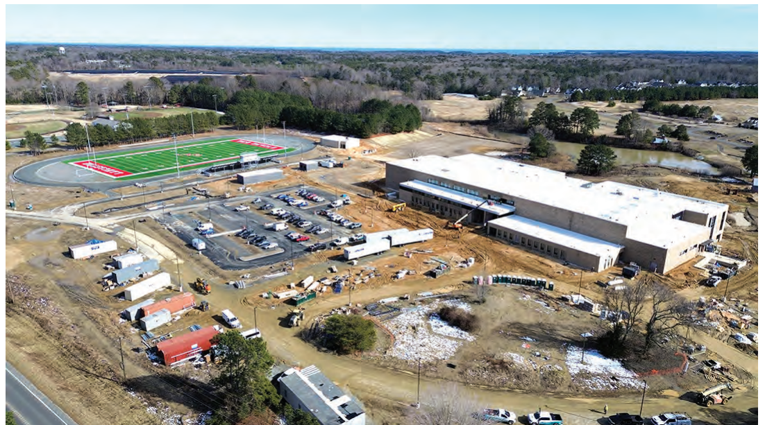
Construction is nearly complete on Lancaster High School, off of Old Saint Johns Road and Irvington Road next to Dream Fields. The new school will welcome students in grades 7 through 12 on August 10. Work on the $75 million dollar project was done by Branch Builds and VMDO. Photo courtesy of Lancaster County Public Schools
