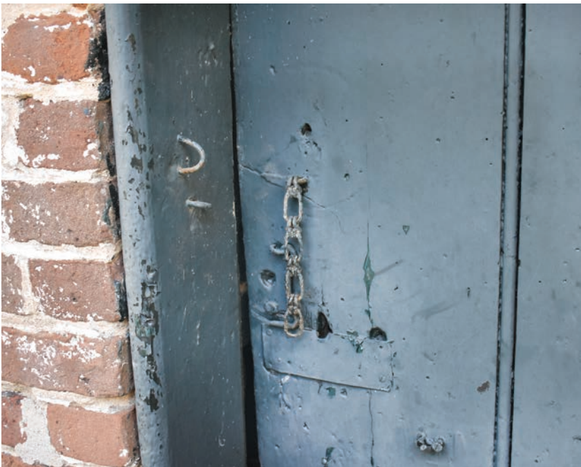
A substantial, well-built door leads to the inside of the dairy well.
