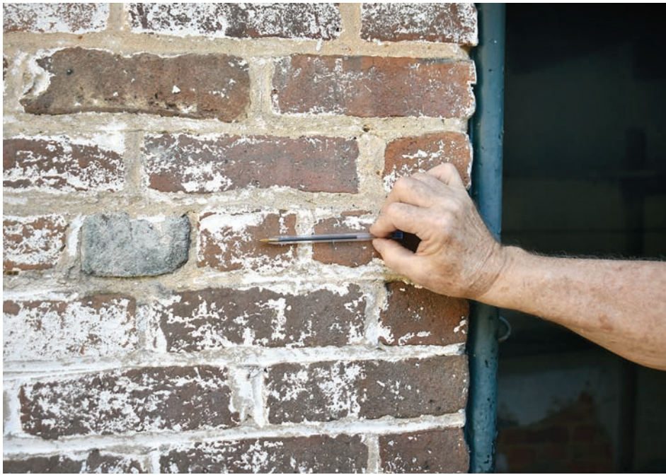
The brick walls are of English common bond pattern where several layers of bricks are laid long ways and then there is a layer turned on end. The brick dairy walls are two feet thick to provide a cool environment inside.
