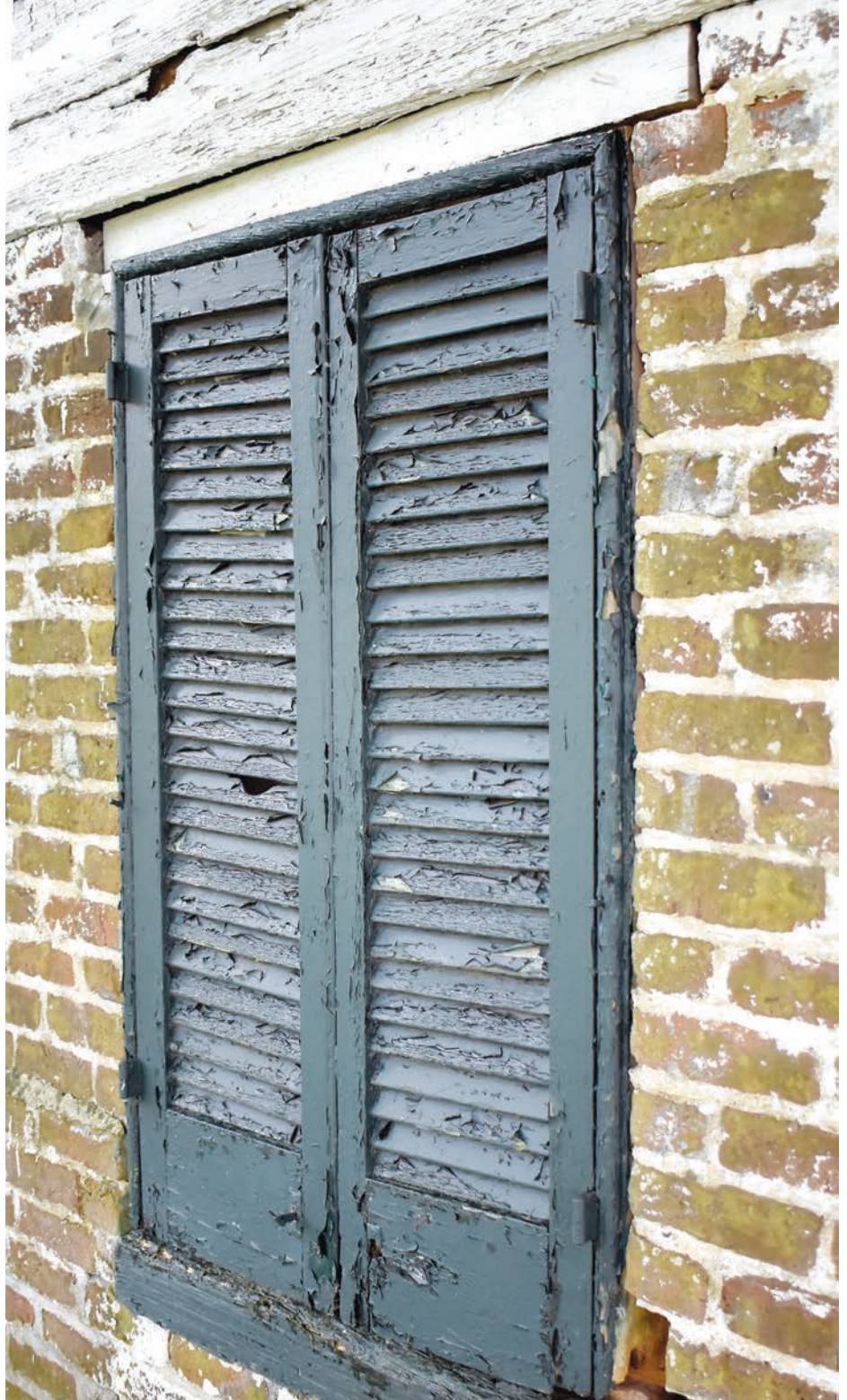
The dairy has two shuttered windows which were unusual for colonial and antebellum dairies. Instead of windows, slots, grilles, lattices, or louvres were used to let air flow through.
